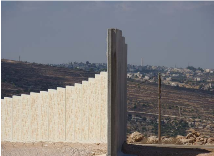
Figure 2: The separation barrier under construction between Walaja and Har Gilo. The barrier is a visual blight on this scenic landscape which the INPA seeks to protect. Baillie-Warren 2010.
